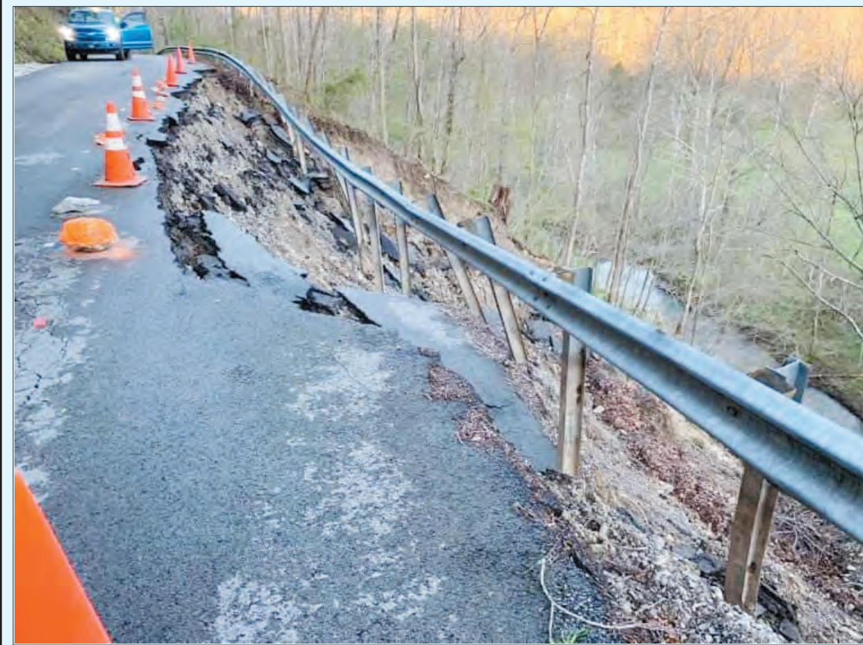
Rockcastle County Judge/Executive Howell Holbrook says there are currently 14 local road slides that he hopes will be repaired soon with the help of FEMA and other funding that he and the fiscal court are applying for every week. This slide on Wildie Road, did not qualify for FEMA funding so Holbrook found grant money through the State Emergency Road Fund. This $92,000 project was approved just this week through an 80/20 state grant and work is expected to begin soon on the project. Funding to repair the other slides in the county are also in the works through different grant applications and Holbrook said work on each slide will begin as soon as each grant is approved.
