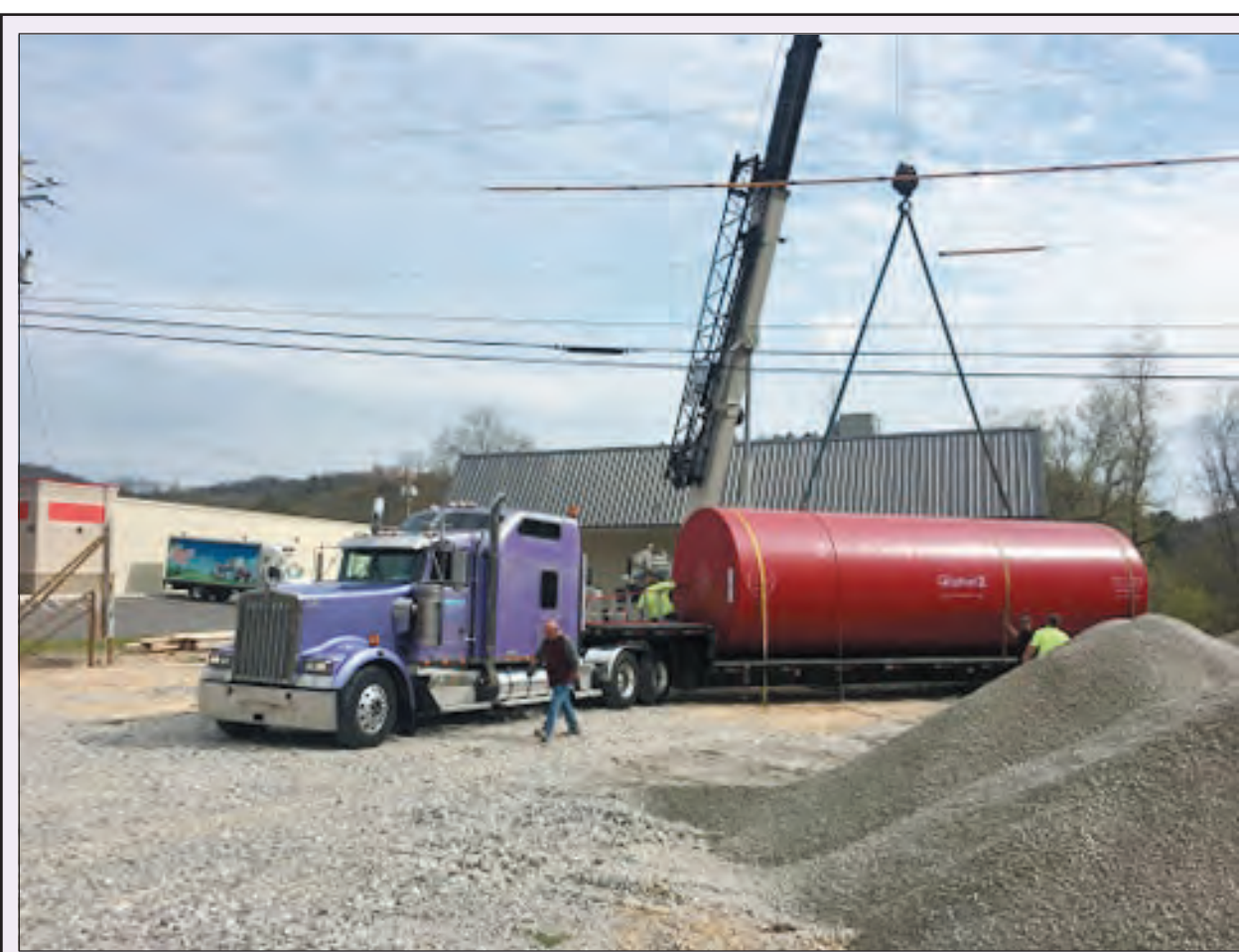
The 20,000 gallon gas tank was placed this week at the new Marathon Station in Livingston and officials say the project is still on schedule. Mayor Jason Medley says the station beside the new Family Dollar Store will be a huge asset to the entire community of Livingston and he is proud to welcome another business to the town. Plans are to open the station to customers this summer.
