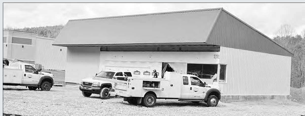
The new Marathon station in Livingston is now under roof and owners are still planning to open for business by Memorial Day of this year. Mayor Jason Medley said the new business will make a noticeable difference to the citizens of Livingston and will provide a convenience that the city has been missing for many years. The station is next door to the new Family Dollar store which opened last year.
