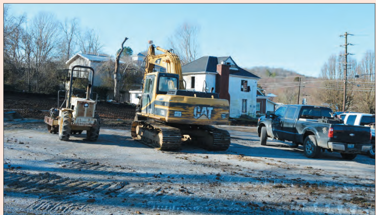
Goff Excavating of Mount Vernon has started the sitework for the upcoming Farmers' Market facility on Richmond Street. The house on the property, in the background, is also being demolished to make room for an entrance and more parking.
