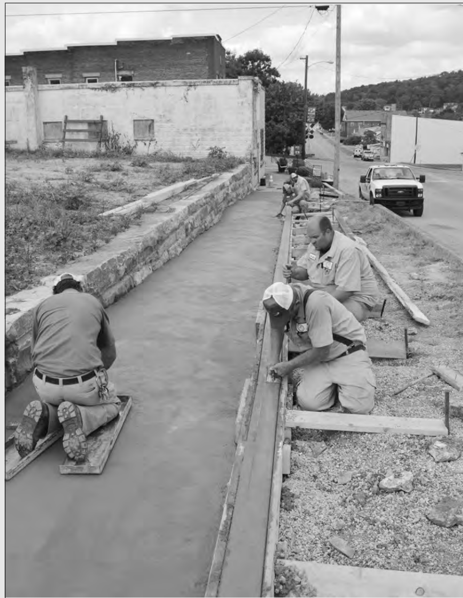
City workers spent most of the day Monday forming and pouring the new sidewalk at the city-owned Sinclair property on the corner of West Main and Richmond Street. Officials are still considering several options concerning the best use of the property but a sidewalk will be required regardless of how the property is finally utilized.
