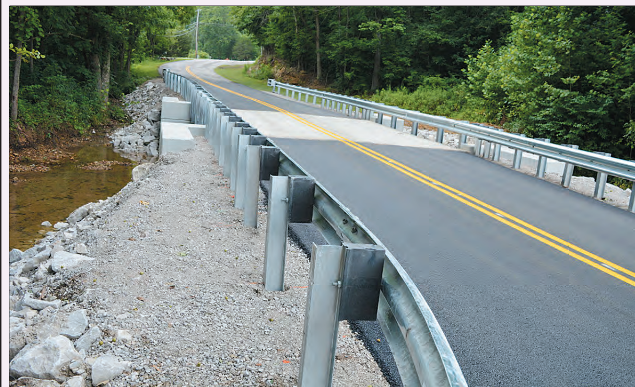
Local residents have detoured the bridge on Highway 1326 since May while a new bridge was underway. The road reopened Tuesday after workers completed the new structure. The bridge is one of many local construction projects in the county that has caused road closures and detours and more construction is expected soon near Renfro Valley since the new TIF District has been established.
