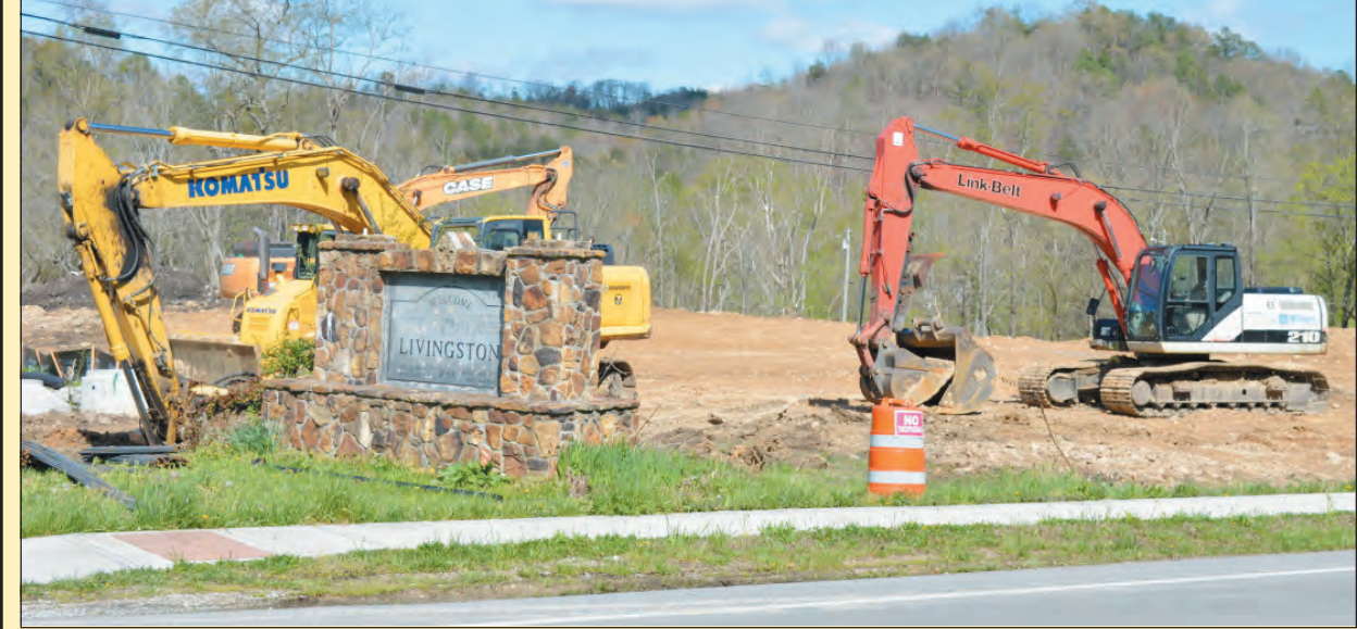
Construction is underway in Livingston for the new Family Dollar Store. Officials expect the store to be open sometime this summer and think it will provide a boost to the local economy. Officials are also negotiating with a Marathon Service Station hoping they will locate on the lot next to the Family Dollar. Mayor Jason Medley said the town is returning to its hayday and the two new businesses will change the atmosphere of the town providing a much needed convenience for everyone.
