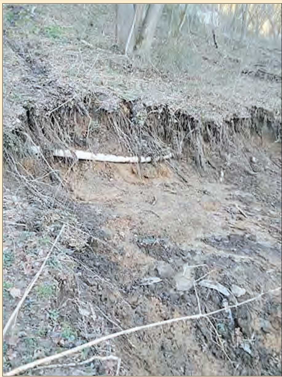
A six-inch water main near Livingston was exposed and broken due to recent mudslides causing 40 customers to be without water for several days. However, crews repaired the line and now Livingston customers are under a boil water advisory until further notice.
