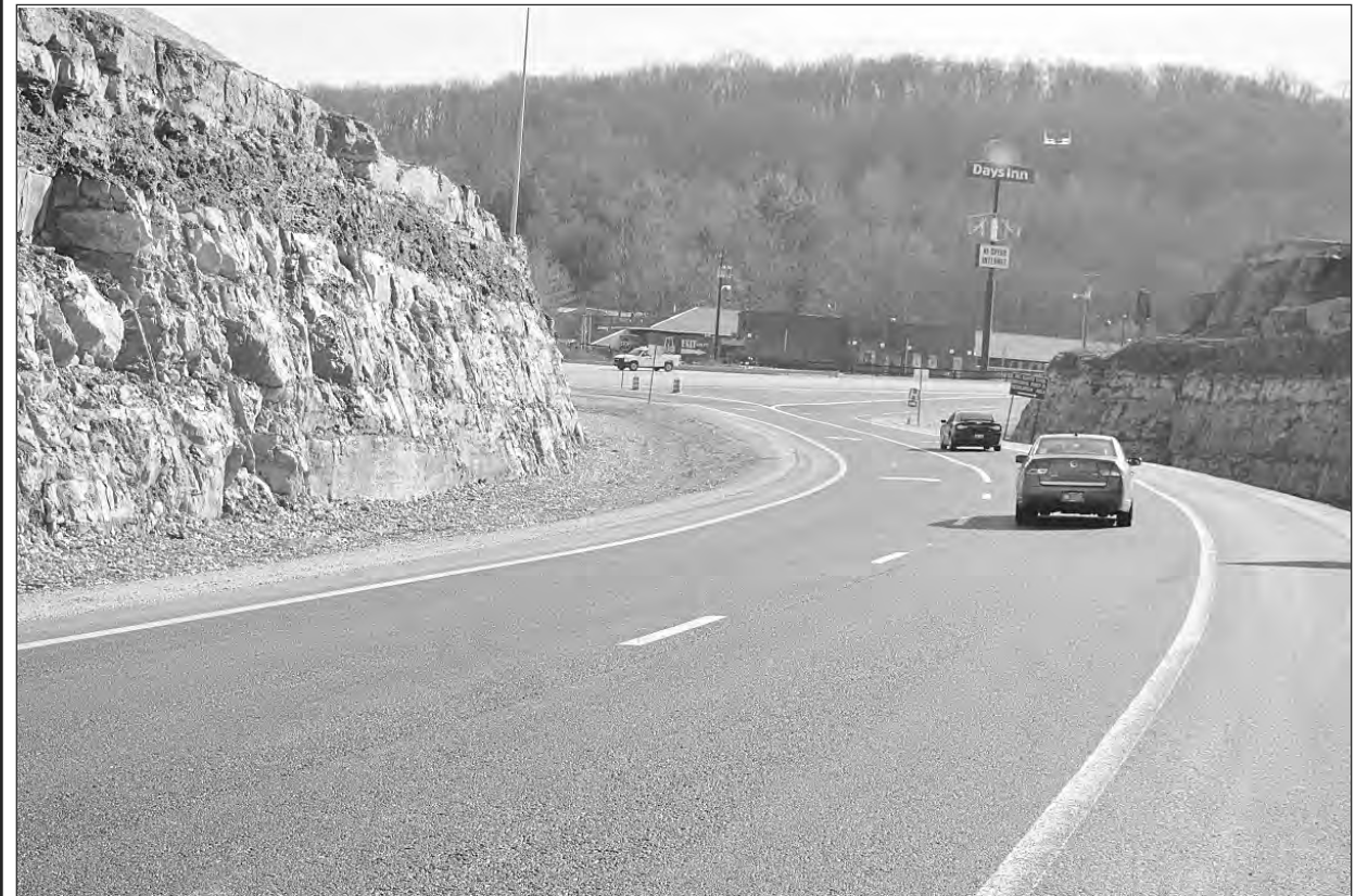
After remaining closed for several weeks, southbound exit ramp 62 in Renfro Valley is now opened. The ramp work is part of the I-75 widening project.
