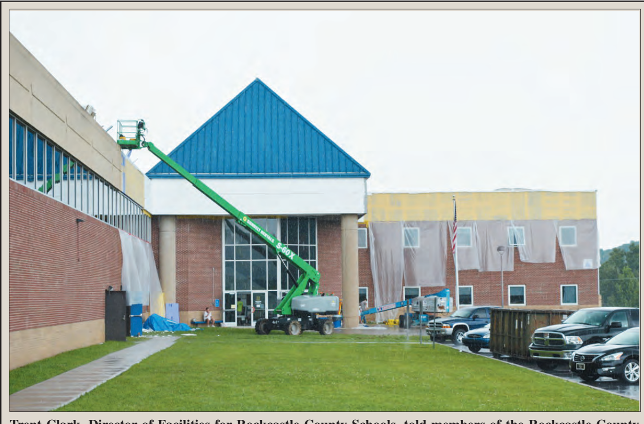
Trent Clark, Director of Facilities for Rockcastle County Schools, told members of the Rockcastle County Board of Education, at their last meeting, that work at RCHS is on schedule and, barring any unforeseen events, classes should begin as scheduled on August 15th. Clark said there were a few slight rain delays in early summer, but the work is still on schedule. Clark said he is working closely with contractors and work on the new front entrance and the heating and cooling systems, as well as other smaller jobs at the school, is progressing.
