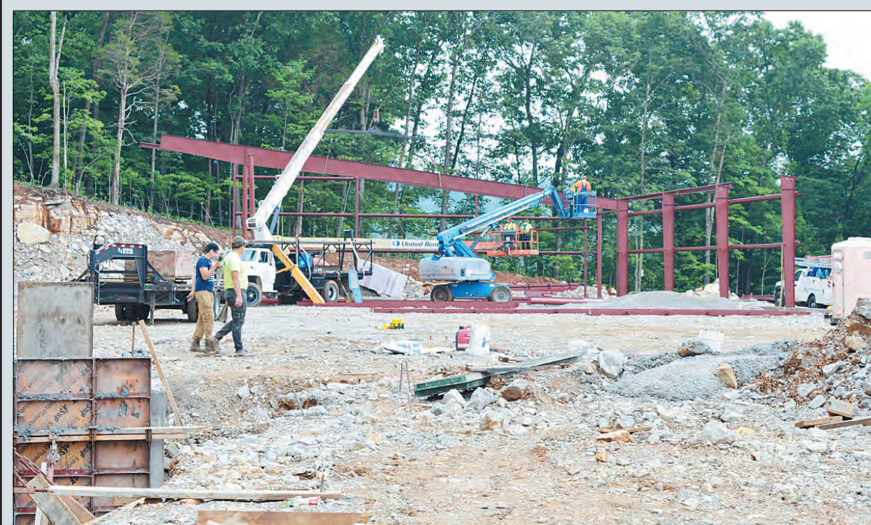
Workers are moving ahead on the new Microfoodery plant, under construction on Richmond Street. The $2.85M project is owned by Karl Krase and partners and actual production is expected to begin on or about August 15th. Owners expect to hire 200 full time employees within two years who will manufacture cheese and other specialty products for sell around the globe.
