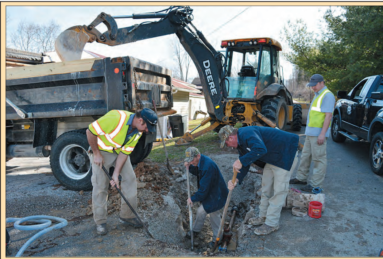
Mt. Vernon City employees jackhammered concrete and dug out a water leak on Richmond Street Tuesday morning. Frank Baker, Maintenance Department Supervisor, said the leak was caused by an older fitting breaking loose and crews were able to repair the leak quickly. According to Baker, only McDonald's was affected by the leak but the restaurant was back in business a few hours after the leak was discovered. Several water lines in Mount Vernon are older and may have fittings that could break loose anytime but Baker said his team are keeping a close eye on areas where lines are older. Baker said this leak had nothing to do with recent temperature changes.
