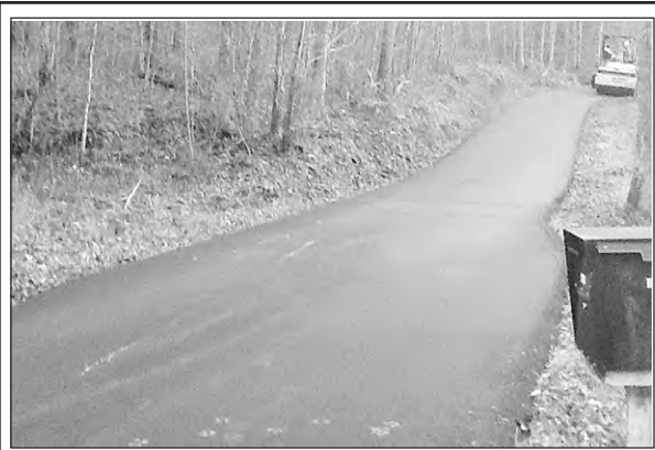
Our freshly paved road here on Piney. First black-top in approximately 20 years. Thanks Michael.
