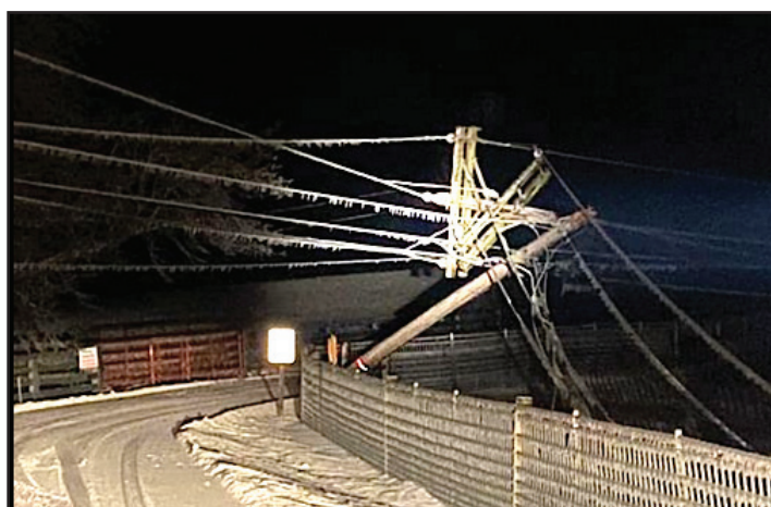
Four utility poles, including the one in above photo, fell in the Jolly Ridge area earlier this week.
